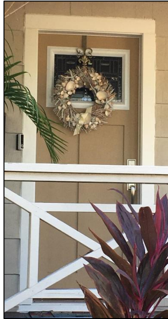
Figure 2: Recently installed door without COA
